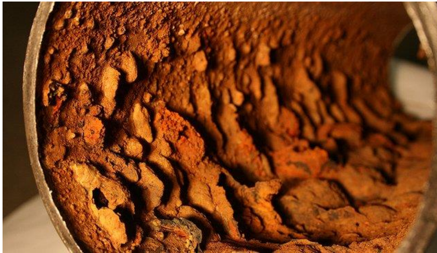
Figure 1.8: MIC corrosion inside a fire sprinkler systems
