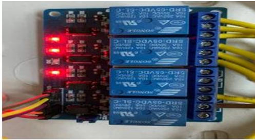
Figure 11: 4-Channel Relay Wiring Termination.
