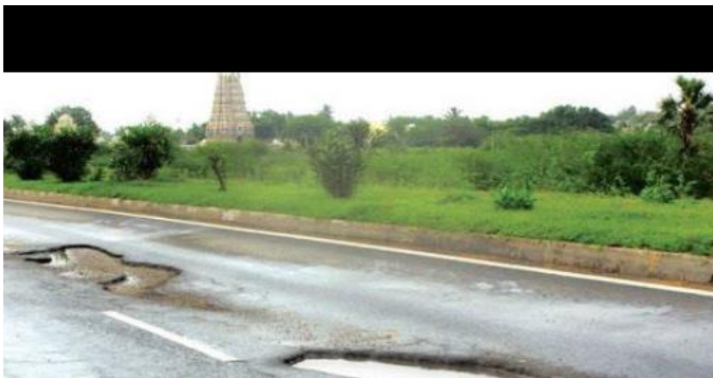
Fig 2: Potholes on highways
