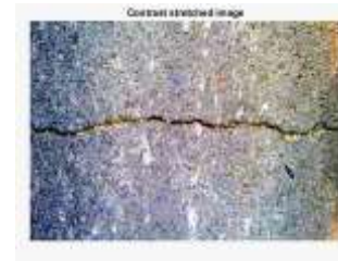
Fig8: Contrast Stretched Crack Image.
